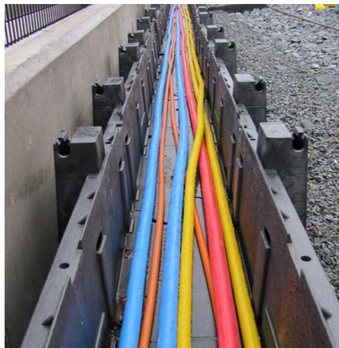
Cable Troughing - Power & Energy
